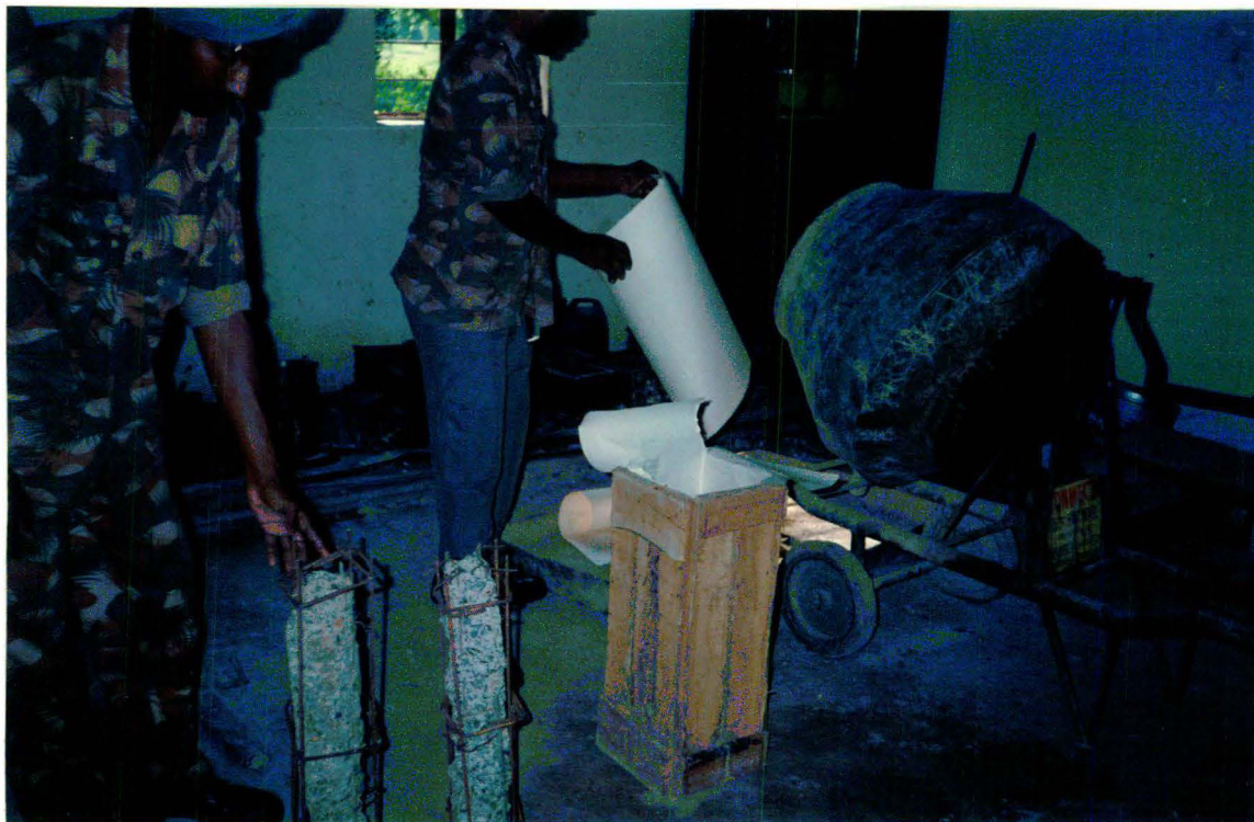
Photograph showing damaged columns and the encasing reinforcement.
