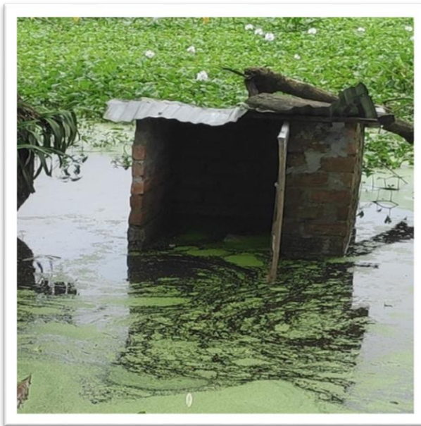
Photo 2: Toilet facilities submerged during flood. Source: The author
