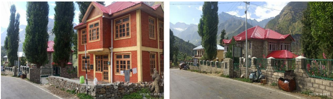
Plate 30: PWD guest house in Sissu area under the Impact of Flood Inundation
