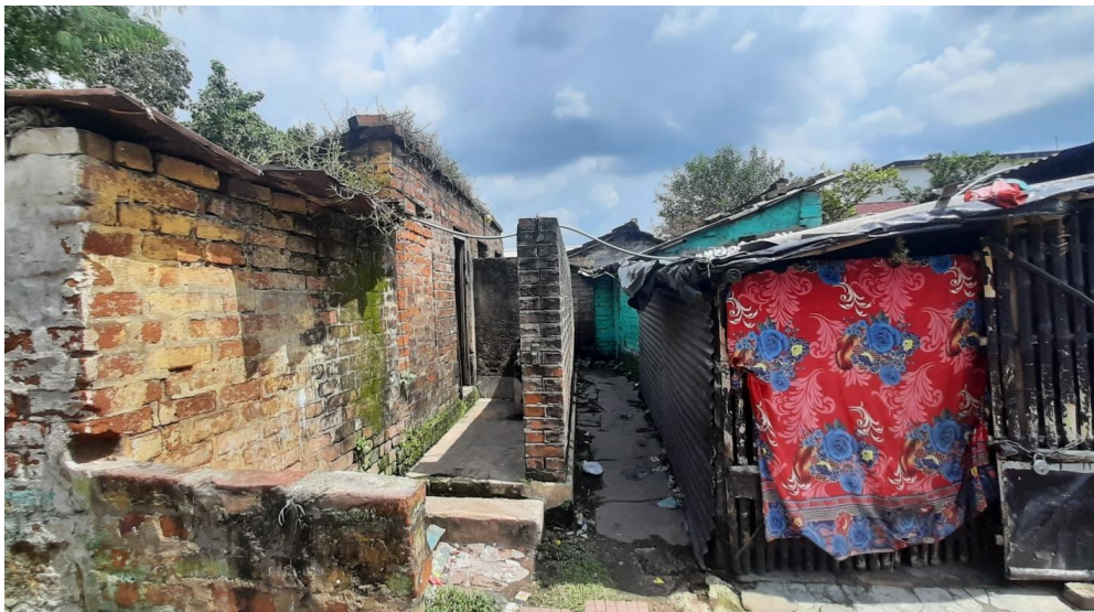
Figure 21: Abandoned Public Latrine Facility in Bastee Line Area
