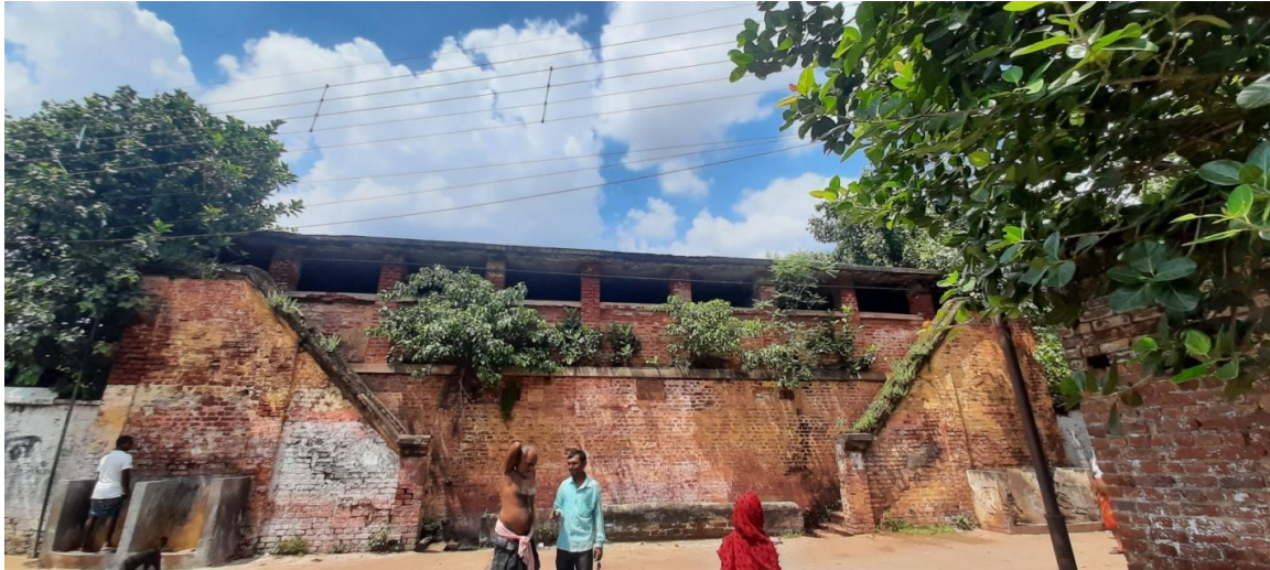
Figure 12: Showing Public Toilet Condition of Reliance Jute Mill Quarters in Bhatpara
