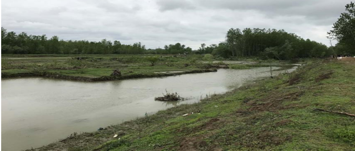
VIEW OF THE FLOOD SPILL CHANNEL AFTER TREE CUTTING AT BEMINA-DURBAL- POSSESSION TAKEN OVER AFTER 27TH OF APRIL-2017 WITH POLICE ASSISTANCE.
