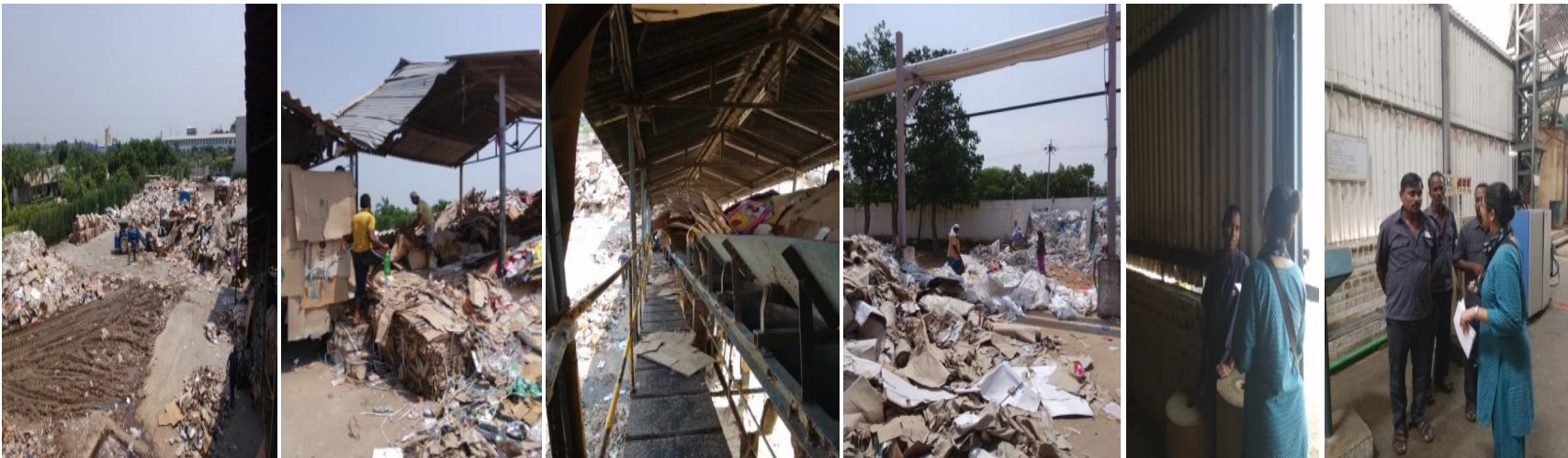
Waste being recycled and sent through belt to form pulp, water is recycled and reused too
