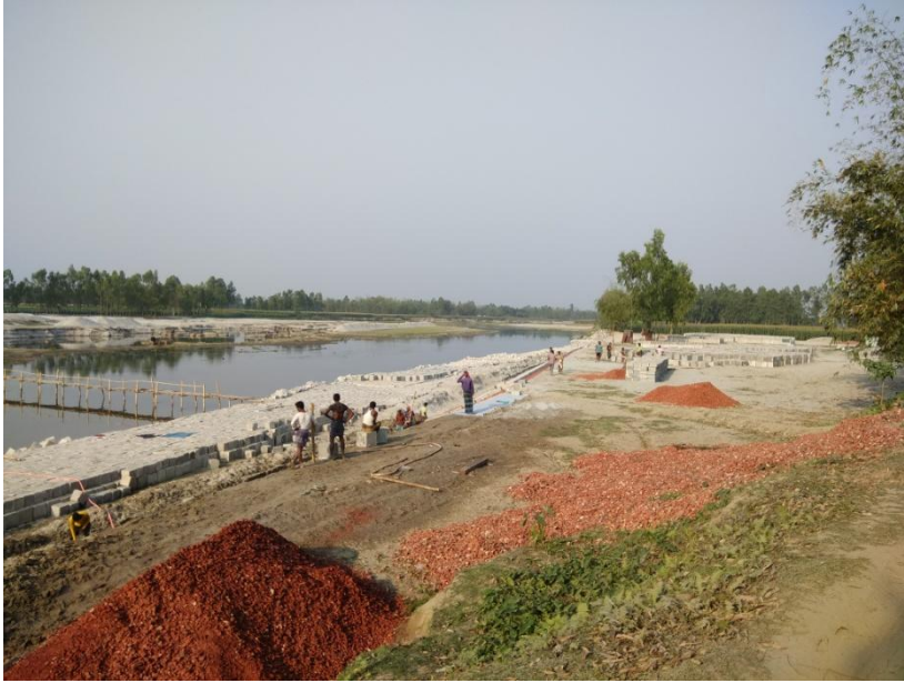
Figure. Development project on river Dharala, former 119 no. Bashkanta Chhit, Patgram, Bangladesh.
