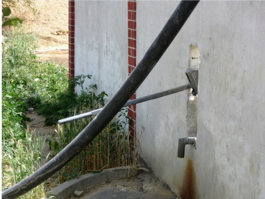
Photo 4: Hand pump in Orgai
