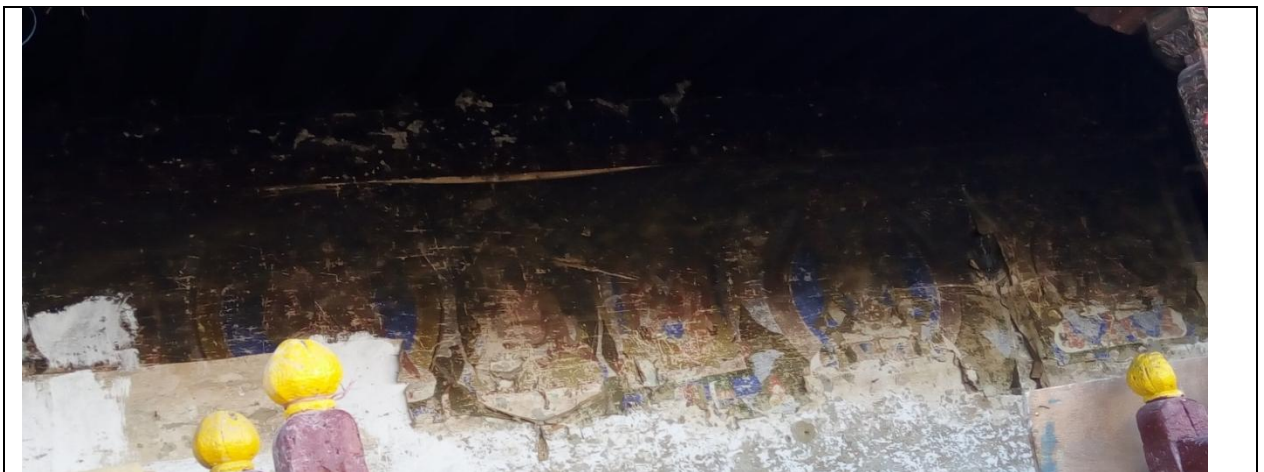
Figure 5: The figure shows the surviving mural painting on the wall of the old library building in a dilapidated condition. (Photo by: Hakhe)
