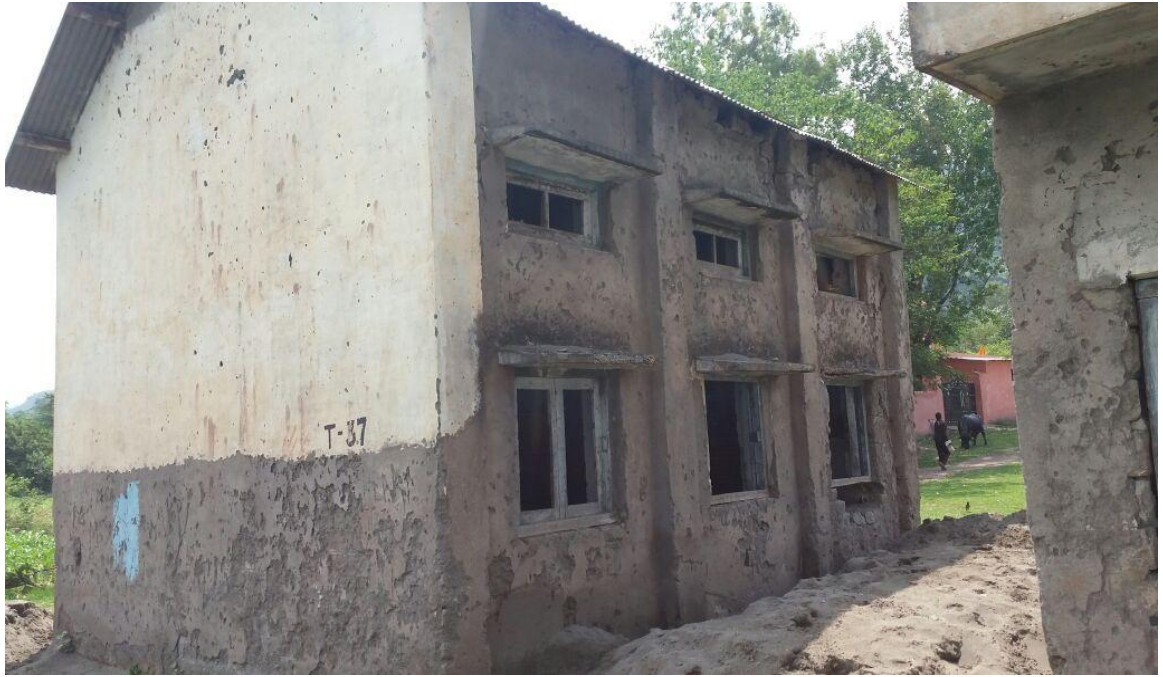
Photo 2: Destroyed school of Jhulaas village by shelling across the borders.
