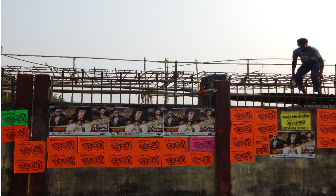
Continuation of construction at Rajtilak Theatre's stage and posters of Rajshri Theatre's play Goonda .
