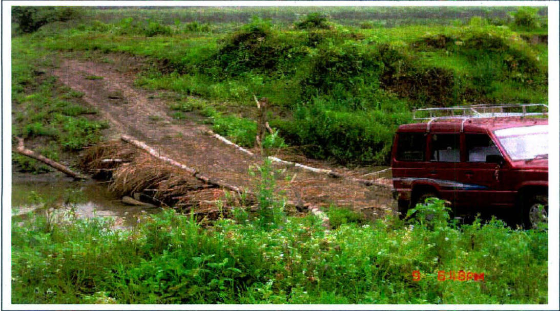
Plate IV.4. Dilapidated culverts in Kaziranga can lead fatalities at any time.
