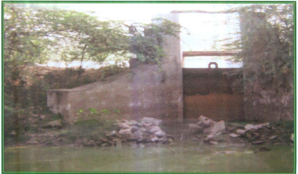
Plate 10. A Sluice gate between two blocks of Keoladeo National Park.
