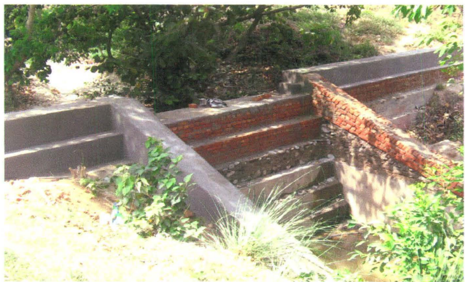
The height of check dams is being raised due to heavy siltation in Kathgarh
