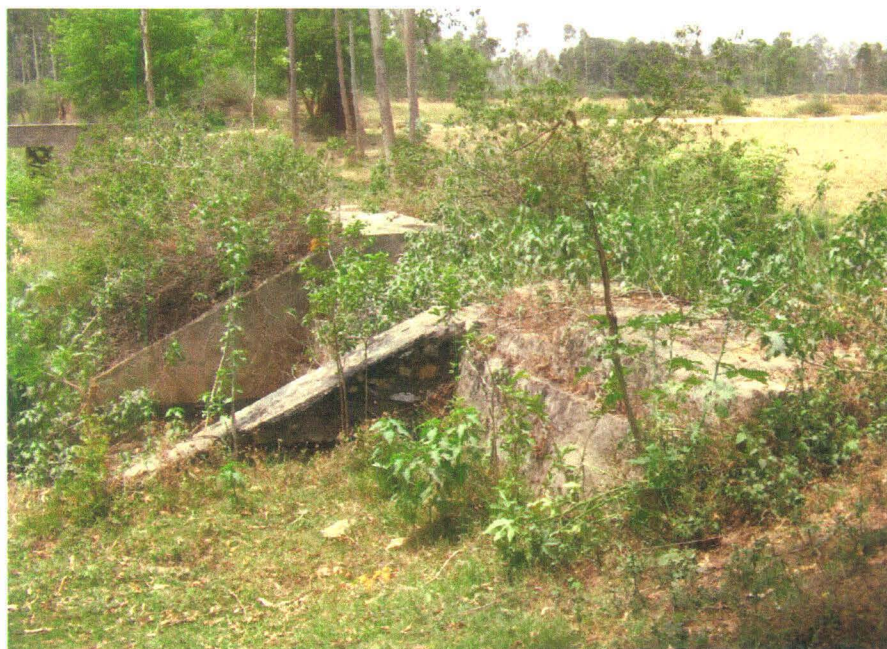
The villagers allege faults in the construction of check dams in Mirzapur
