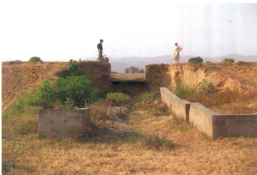
Structures built in the commons have all got damaged
