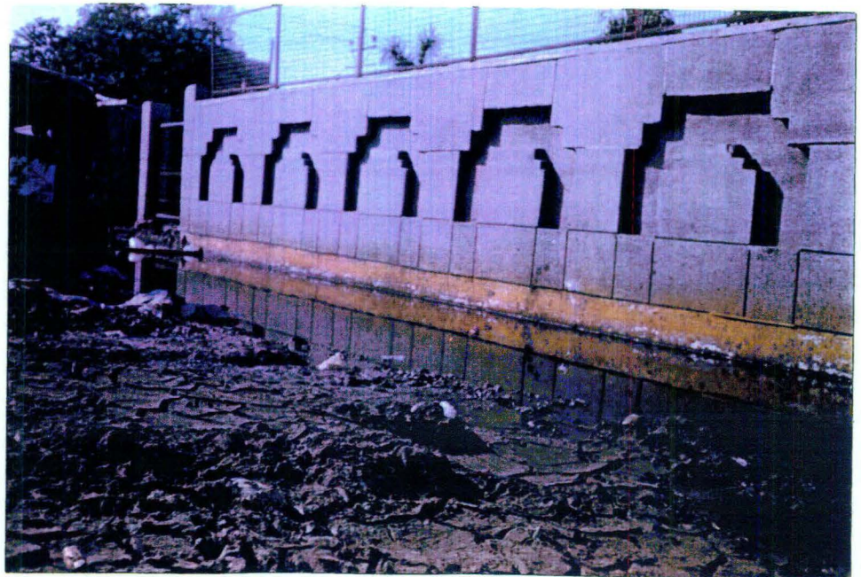
Roadside dumping of sludge in Block B, Wazirpur
