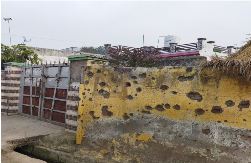
Splinter marks on the wall of a house in village Suchetgarh (Photo by Author)
