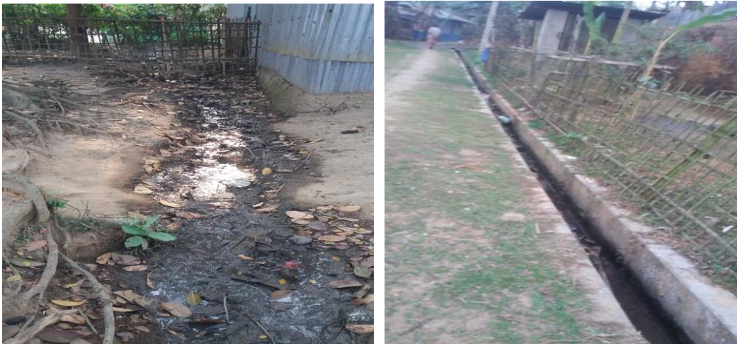
Pic 4.6: Drainage system at labour line of Meghlibund (Left) and Durgabari (Right) tea estate
