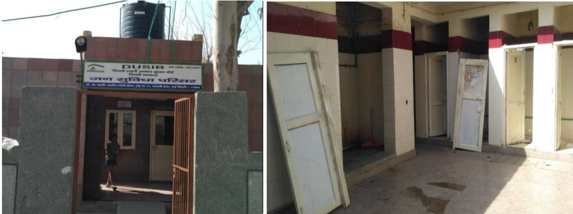
Figure 6.3: The picture (left side) showing that a girl walking out of the pay-per-use toilet which has no water supply and caretaker's room is locked. And the other (right side) picture showing that the newly constructed pay-per-use public toilet block is under maintenance and made up of lower quality materials resulted into detachment of doors of latrine blocks in Rajiv Camp settlement, Punjabi Bagh. Photo captured by the Researcher.
