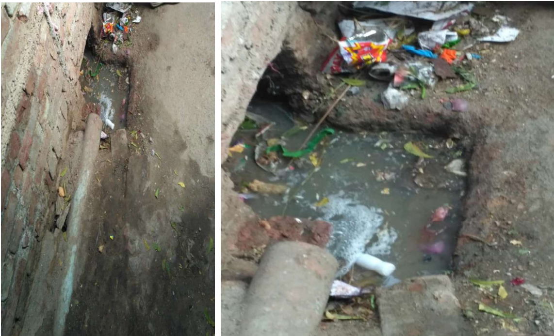
Figure 5.2: Left hand side photo shows a piped discharge in open drain. Right hand side shows excreta are floating in open drain. As drains are open, during monsoon due to water stagnation
