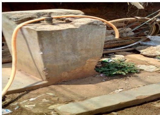
Plate 1: Condition of the Public Stand Post (Bhimpur Area, Site 1)
