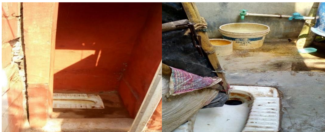
Plate 9: Condition of Congested Toilet (Bhimpur Area, Site 2)
