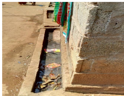
Plate 12: Condition of Drainage facility (Bhimpur Area, Site 1)
