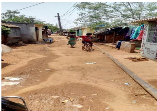
Plate 28: Kutchra Road condition in Bhimpur Area, Site 2
