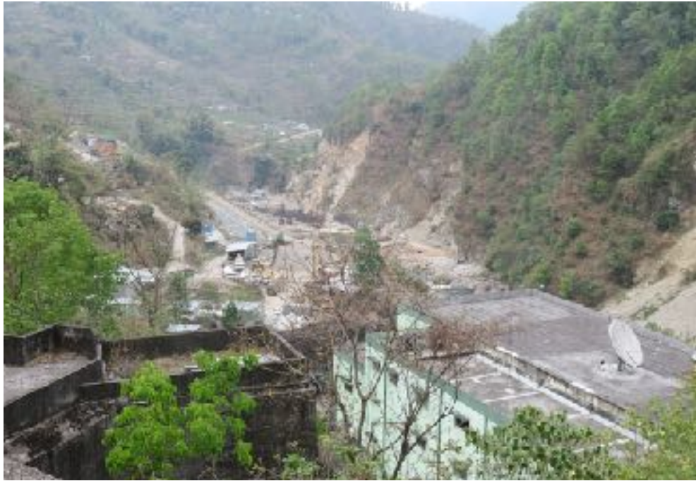
Source: Construction of a hydroelectricity project at the Sikkim-Bengal border. Photo by author at the West Bengal-Sikkim border, dated 10/4/2018.
