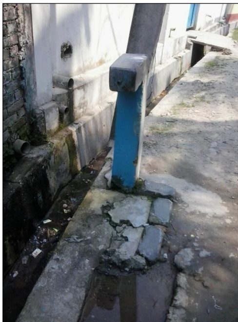
Plate-4.1: Although blue-painted stand-posts are functional, broken platform and absence of stop-cock are serious problems in SMC.
