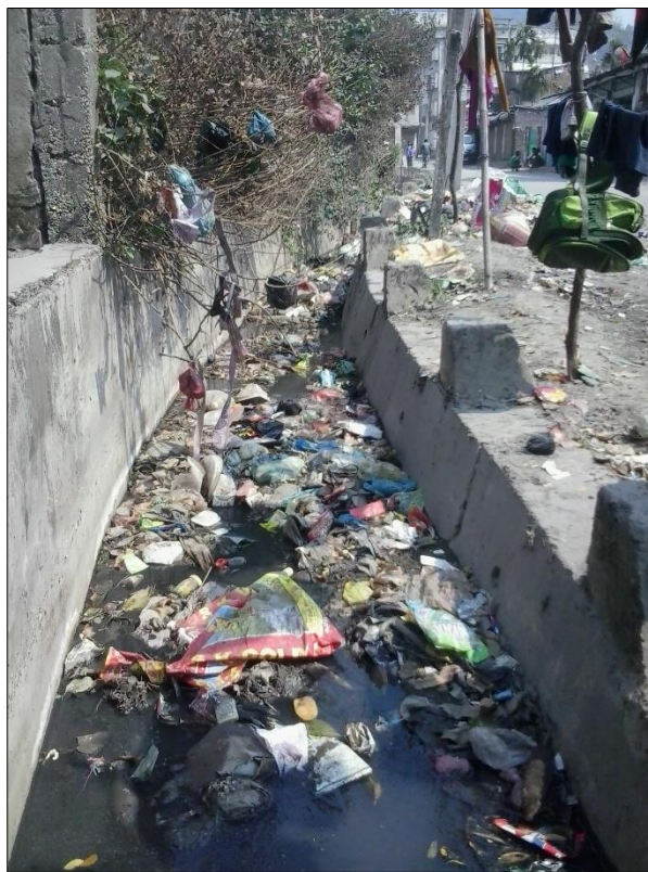
Plate-4.20: Waste water outlets empty into garbage-clogged main drains, Jaigaon
