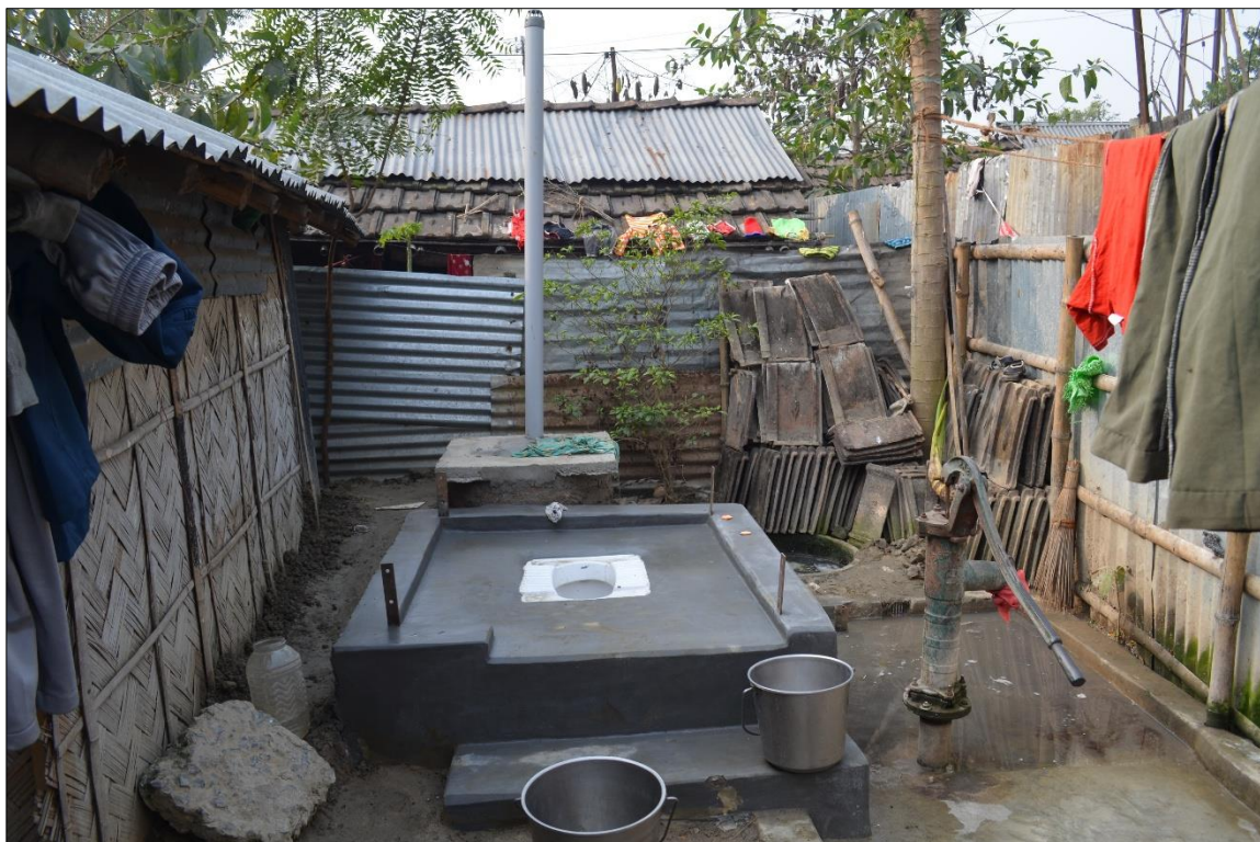
Plate-4.11 EBM: A Ventilated Pit Latrine with Slab under construction. Although a source of water, i.e. a hand pump is visible, walls and roof of the latrine are yet to be constructed.
