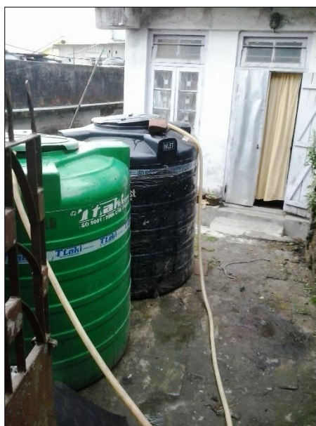
Plate-4.16: Stored water in tanks, Kurseong
