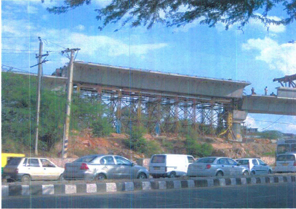
Metro Rail bridge connection on ridge- Mehrauli area of South Central Ridge.
