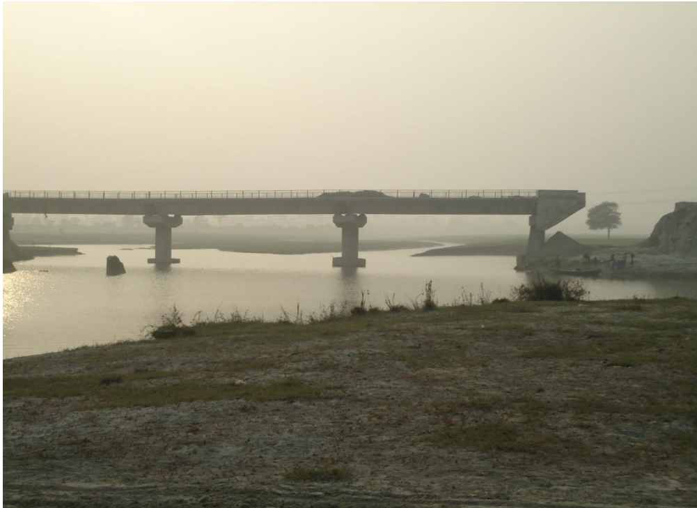
The damaged bridge
