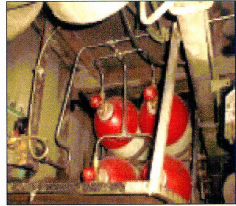
2(c)Too rigid/Unsupported piping
