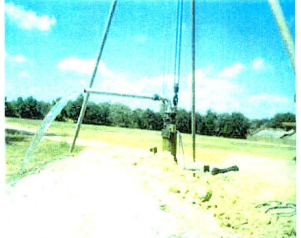
Site 2 (JNU 2) groundwater exploration showing 28,938 liters per hour discharge. The depth of drilling was 182.92 meters with four prominent fracture zones
