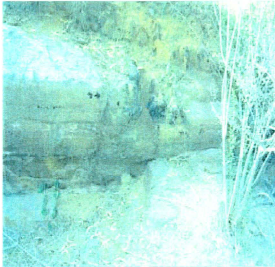
Seepage from the fractured quartzite in RR Hospital Area
