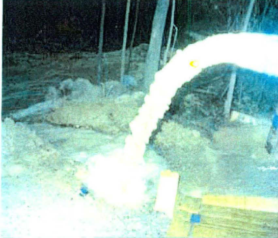
Site 3 (JNU 3) groundwater exploration point showing 34,125 liters per hour discharge. The depth of drilling was 164.63 meters with five prominent fracture zones
