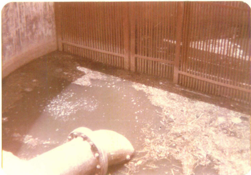
STATION NO. 1 OF PARTIALLY TREATED SEWAGE
