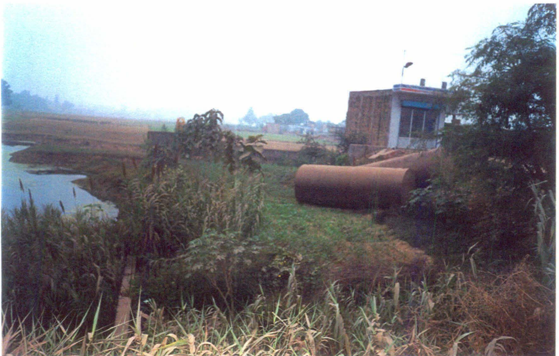
Plate 8: Lifted petrol tanks show the severity of 1998 floods along NH 29. Natural Tal created due to flood is visible on the left.
