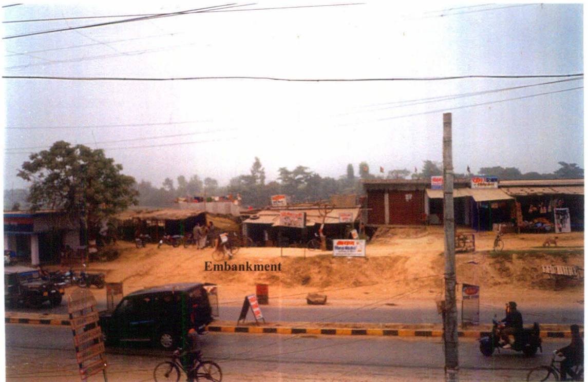
Plate 9: Presence of Gumati (small shop) and households attract more rodent population, which burrow and weaken the embankment along the NH-28.
