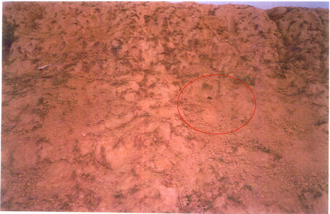
Plate 4: Rat holes are responsible for the seepage and weakening of the embankment-2 during monsoon season.
