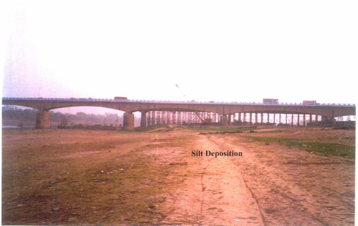
Plate 10: Siltation in riverbed of the Rapti near Harbird bridge does not provide enough room to flood water during monsoon season.
