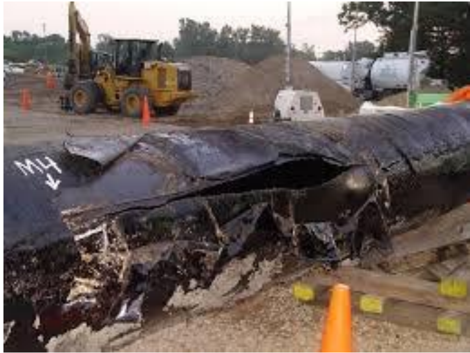
Figure 2: Ruptured Pipeline Responsible for Kalamazoo Spill
