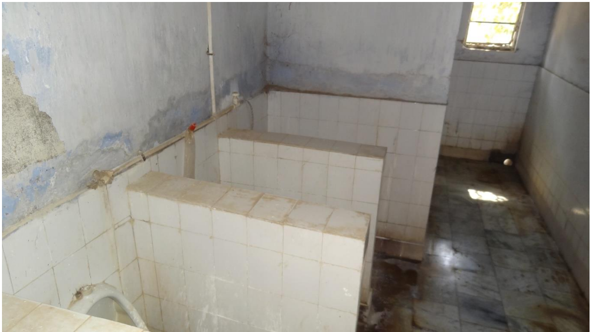
Condition of Men Toilet, District Office, Lohardaga
