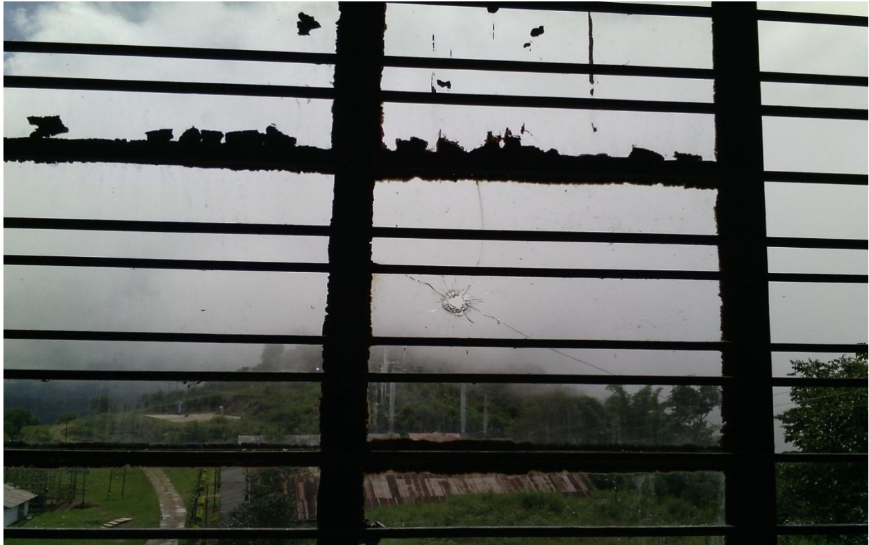
Image 6.2: A classroom window of the KPA damaged during crossfire
