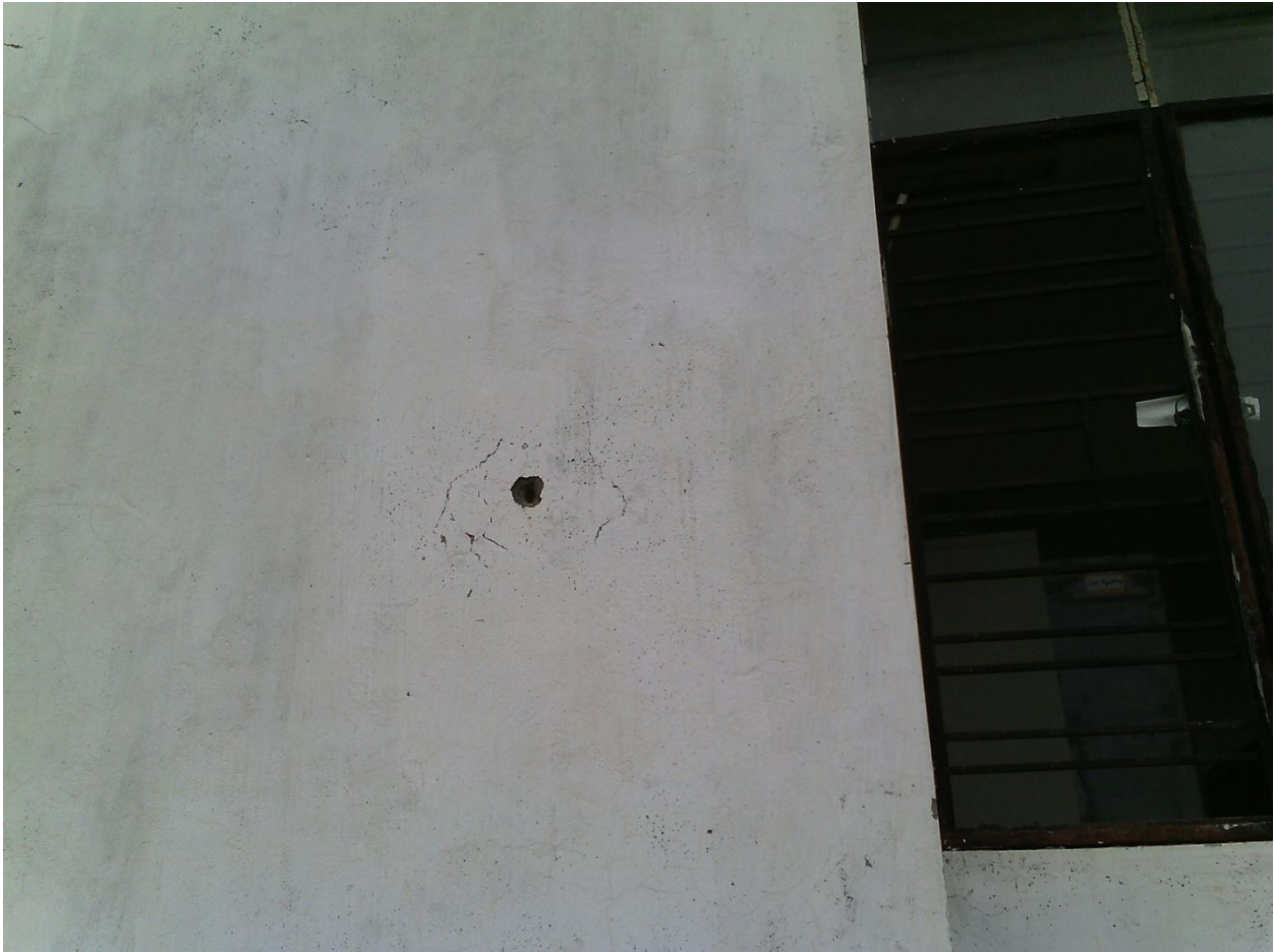
Image 6.1: Bullet mark at the college building caused during crossfire
