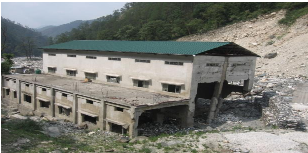
Power house of a project affected in Assiganga flood of 2012 of 2013 (Uttarakashi, 29.6.14)
