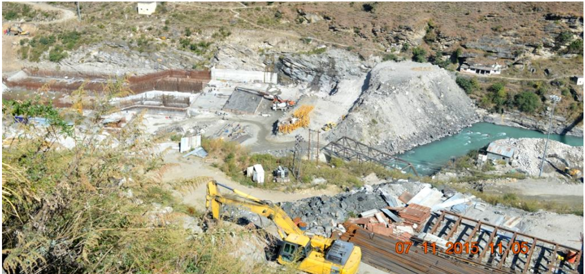
Diverting the River: Cofferdam of NTPC project on Dhauliganga river at Tapovan, can be seen as diverting the river. Also evident is the change in the landscape.
