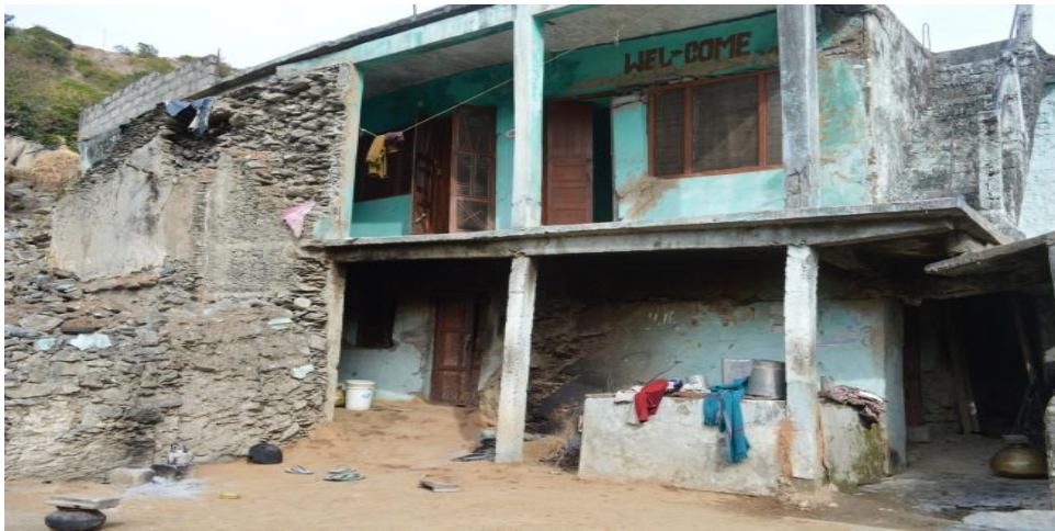
Crumbling houses. The walls and roof of this house with the sign of 'welcome' are coming off, but still people keep living in it (Village Nakot, 19.12.14)
