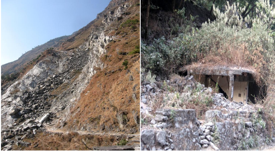
When the mountains subside helplessly: Landslide in Khela grazing ground since February 2009, known as Chetual Dhaar and landsink in Ela tok of Shakuri Village due to tunnel leakage in Dhauliganga project (pictures dated 21.12.13), both in Dharchula district.
