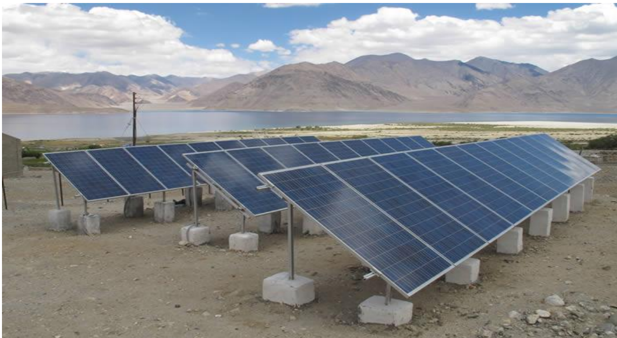
Figure-18: Solar Power Plant at Changthang.
