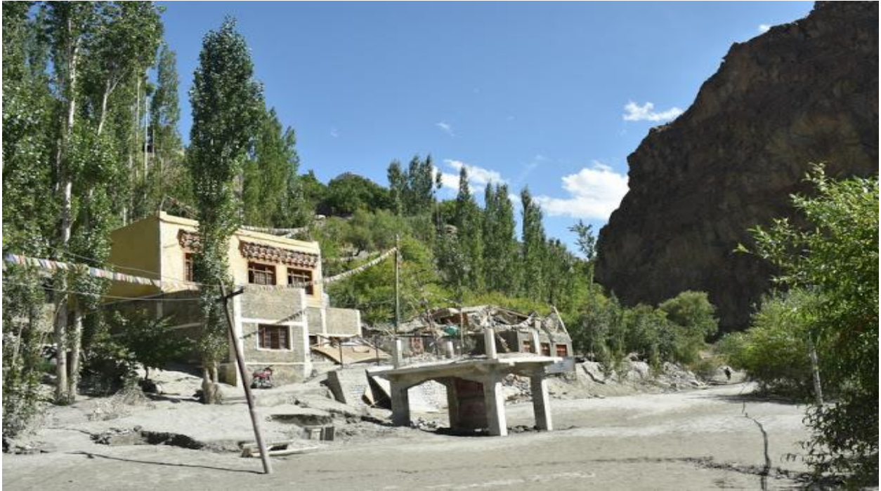
Figure 8: The destruction caused by a flash flood at Bema and village submerges into sand dune after water level went down.
