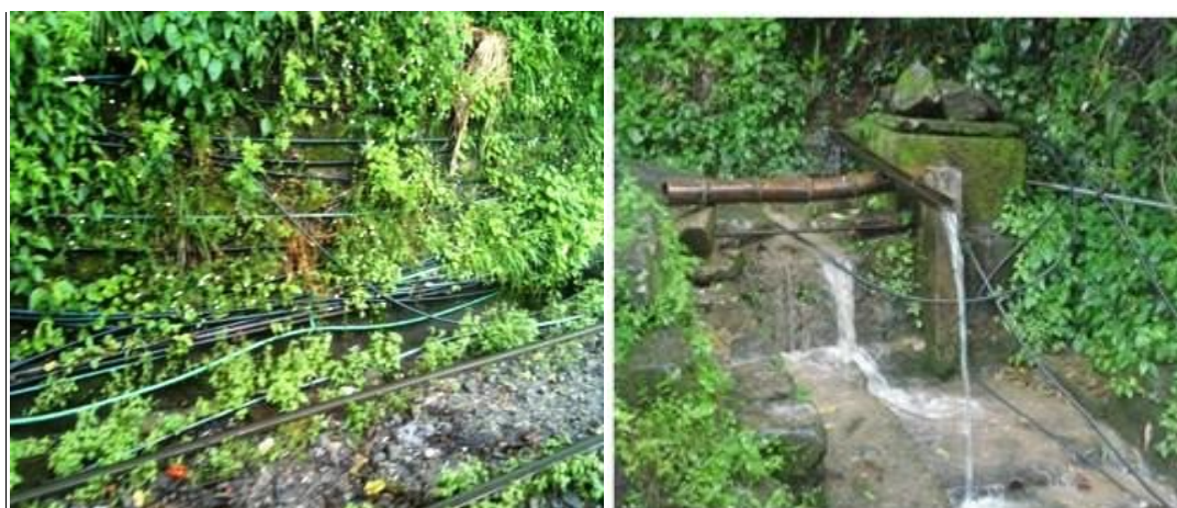
Plate 3.3 Piped Water Supply and Spring Water in Tea Gardens of Darjeeling
