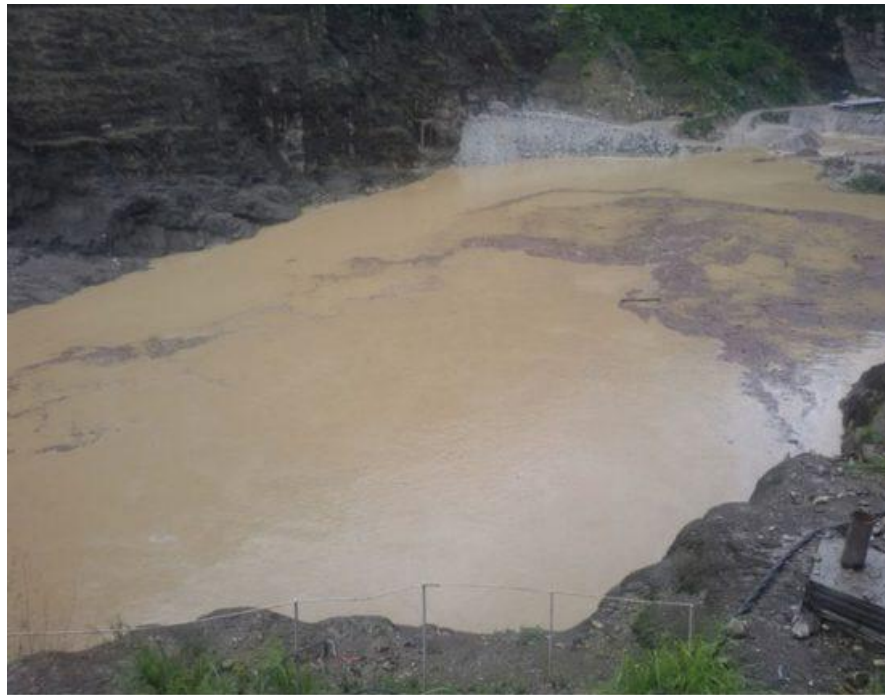
Picture 15: Punatsangchhu-II construction site was flooded due to overflow of Cofferdam
