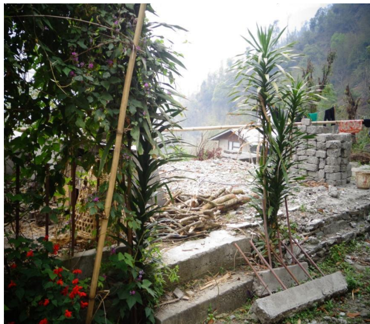
Picture 46: House developed cracks due to blastings in the project site and later it collapsed
