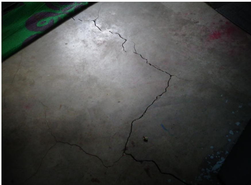
Picture 48: Cracks in the house due to rigorous blastings in the project site
