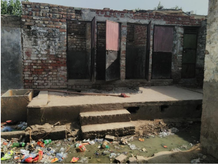
Plate No. 13 – Filthy Washrooms – For Common Use
