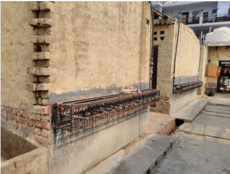
Plate No. 11 – Metered Water at Kapashera at Worker's Residential Units
