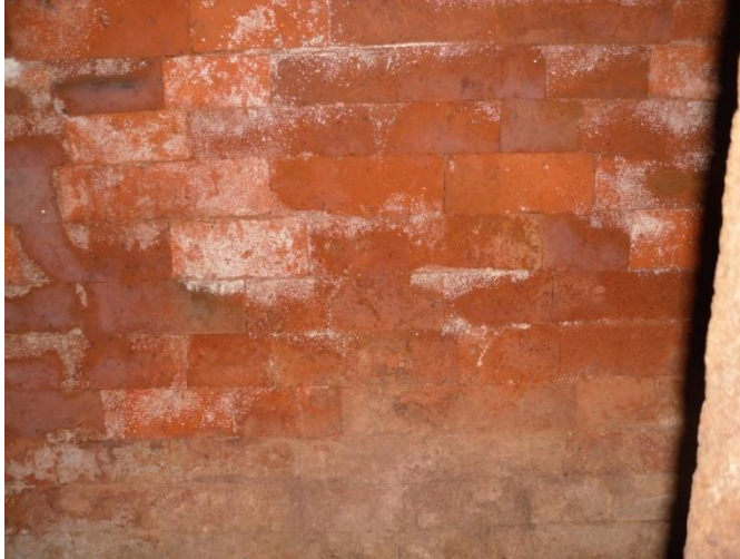
Figure 3.8. One of the walls of the shrine of Monastery I that exhibit the effects of chemical wash.
